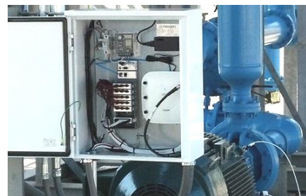
Figure 7. Sample data acquisition hardware cabinet
